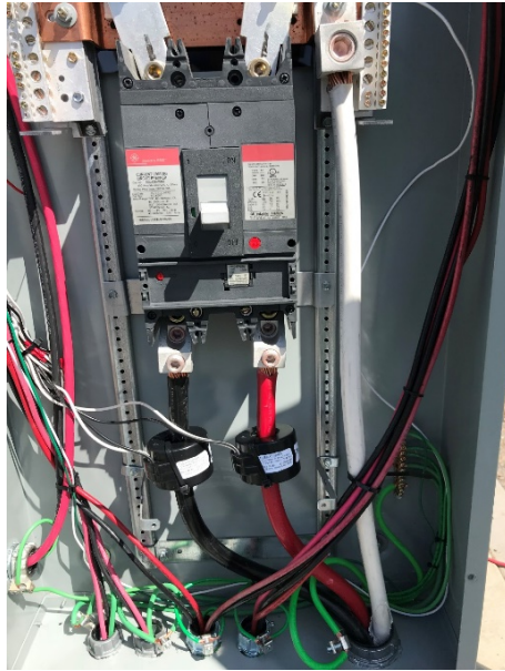
Figure 15: Open Breaker Panel Showing TMS CT Connections
