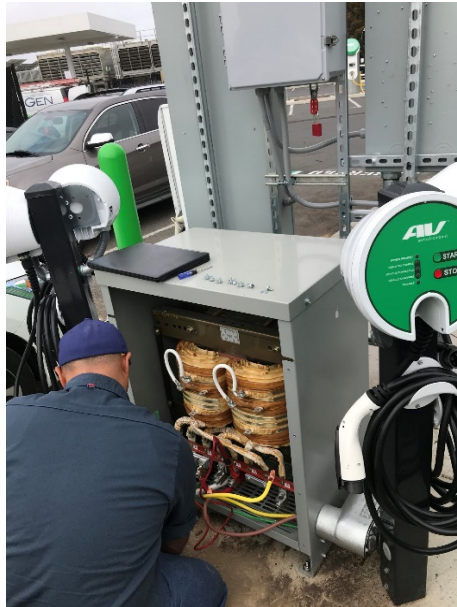
Figure 16: Foreground 75 VA Transformer and Electric Vehicle Supply Equipment
