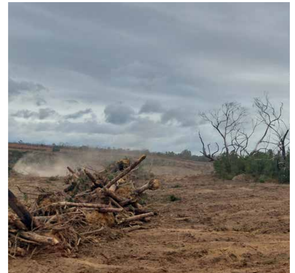
Image right: Forestry clearing is underway across KI. KILB staff are working with landholders and contractors to explain the implications of clearing forestry on the water resource, including the ability for neighbours to build dams.
