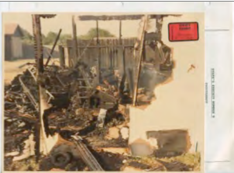
Photo 2: Overall fire damage to the shed at Graf fire (Exhibit 9)
