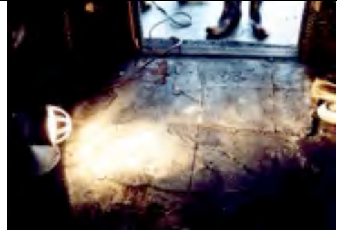
Photo 7: Floor burn pattern to vinyl tile and front door threshold in the hallway of the Willingham fire.
