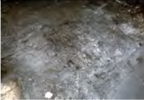
Photo 6: Floor burn patterns to vinyl tile in the Willingham fire.
