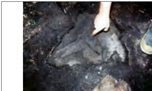
Photo 16: Burn damage to floor in the northeast bedroom of the Willingham fire.
