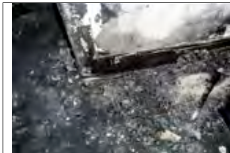
Photo 3: Low burning to floors and baseboards at Willingham fire.
