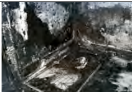
Photo 4: Low burning to floors and baseboards at Willingham fire.
