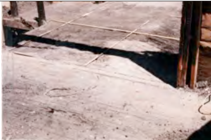
Photo 8: Floor burn pattern to hardwood floor in the living room of the Souliotes fire.
