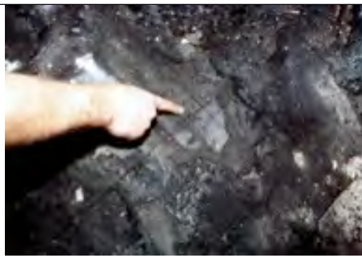
Photo 17: Burn damage to floor in the northeast bedroom of the Willingham fire.
