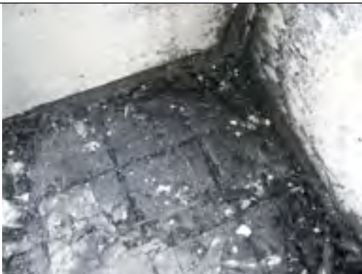
Photo 13: Low burning to baseboards and vinyl tile in burn cell #4.
