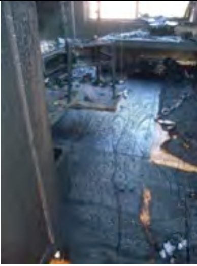
Photo 19: Floor burn patterns to plywood sheeting of burn cell #3.
