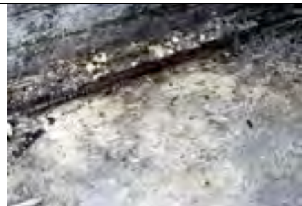
Photo 5: Low burning to floors and baseboards at Willingham fire.
