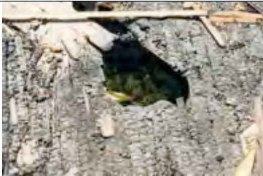
Photo 18: Hole burned through the living room floor of the Souliotes fire.
